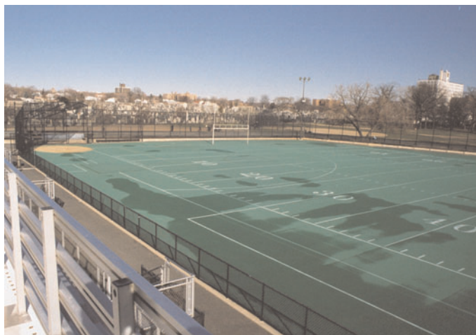
A view of a newly constructed synthetic field at Erasmus Hall High School in Brooklyn.
